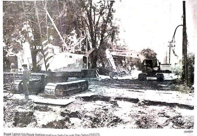
Proyek. Caption foto Proyek frontage road ruas Delta Sari arah Waru Selasa (12/12/23)
